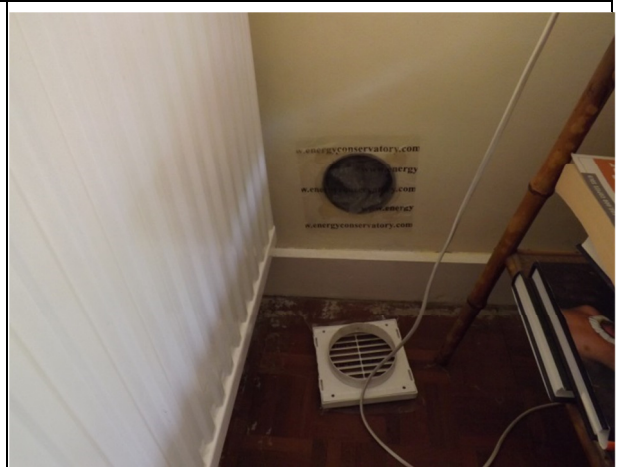
Extract fan upstairs temporarily sealed for duration of testing
