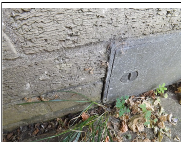
Leakage through gaps around access hatch at base of front wall
