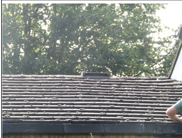
Open ridge vent from original heating to next door making co-pressure testing problematic
