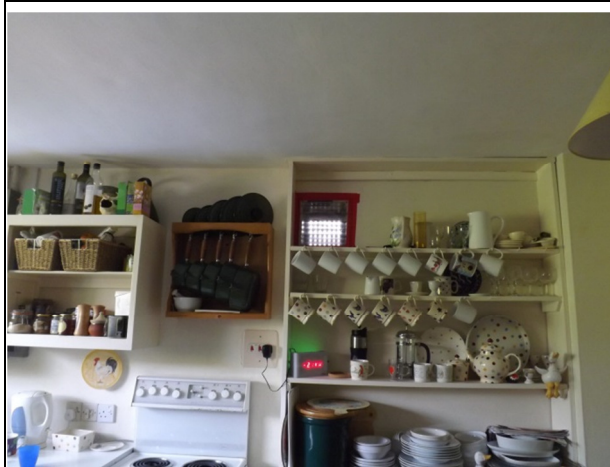
Airbrick in kitchen, largely sealed by resident, temporarily sealed for the test
