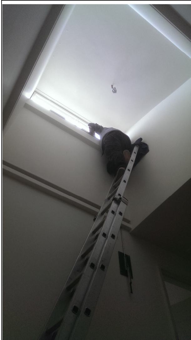
P8) Adjustments being made to dormer window and electric closer to achieve an effective seal. By far the most significant leak identified
